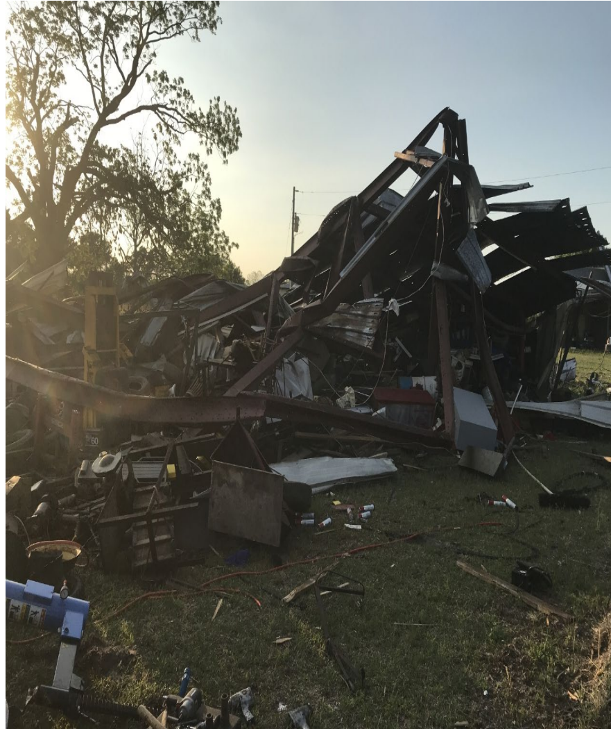
EF3 Damage Livingston, SC – 4/13/2020 Estimated Maximum Winds: 140 mph
