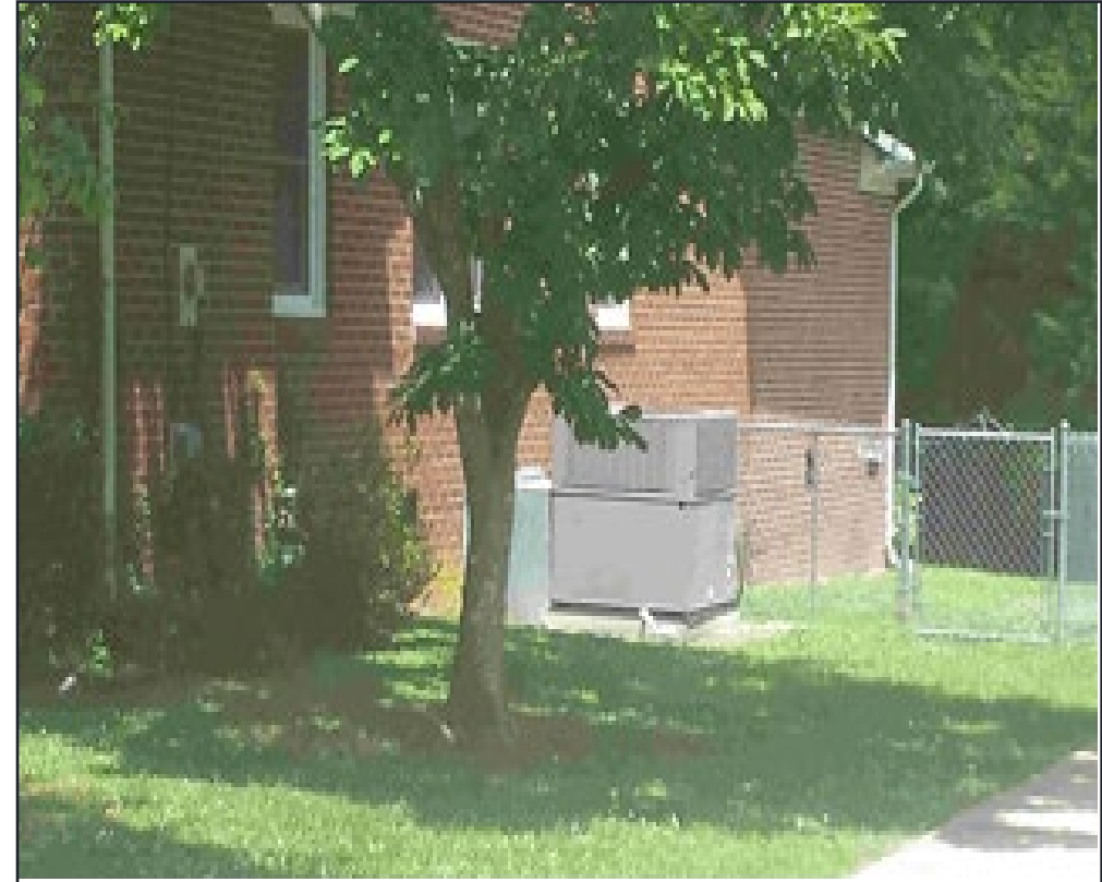
Repetitive Loss Area 3 – HVAC unit on ground
